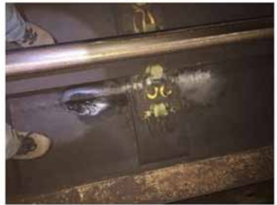
Wet spot on trackbed
