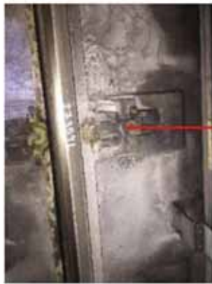
Corrosion of clips
